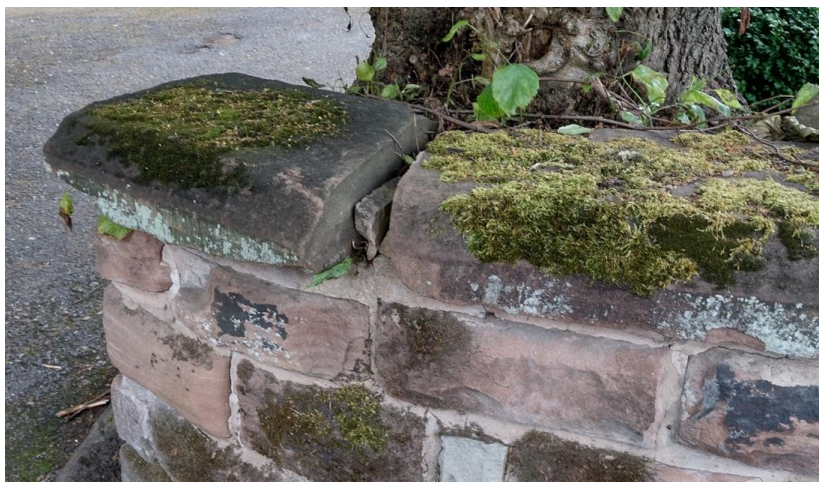
Image 2: Photos of base of protected trees, site access and boundary wall – taken 13 th July 2023.
